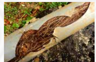
Tree roots can intrude on wiring in rigid PVC conduit
