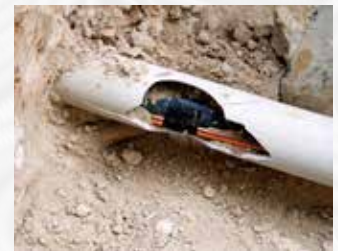
Rigid PVC conduit may be broken by impact
